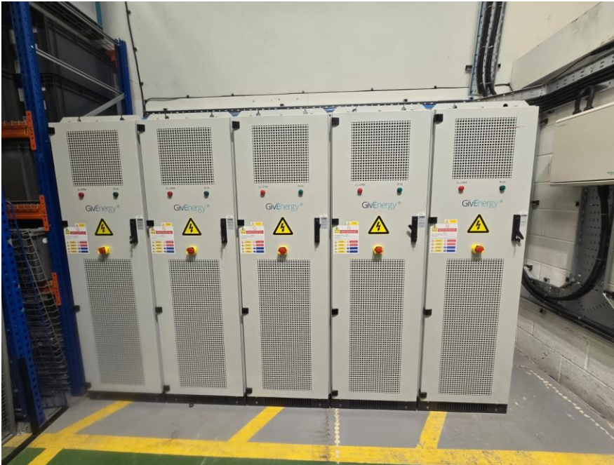
345kWh Battery System at Winchester & Eastleigh Resource Centre, using Lithium Iron Phosphate chemistry:
