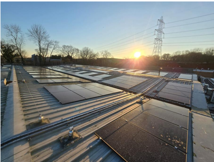
277kWp Solar PV system at Winchester & Eastleigh Resource Centre:
